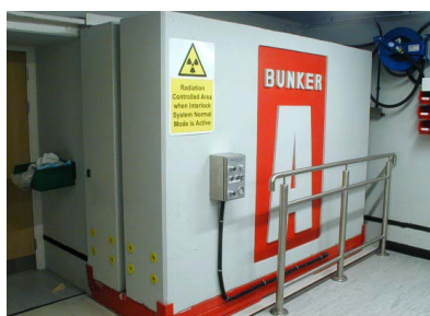
Radiation shielding concrete door to Bunker A in SCAPA
